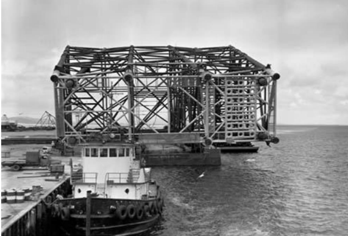
Figure 1-3 One of the Kingfish Steel Piled Jackets being transported to its installation location
