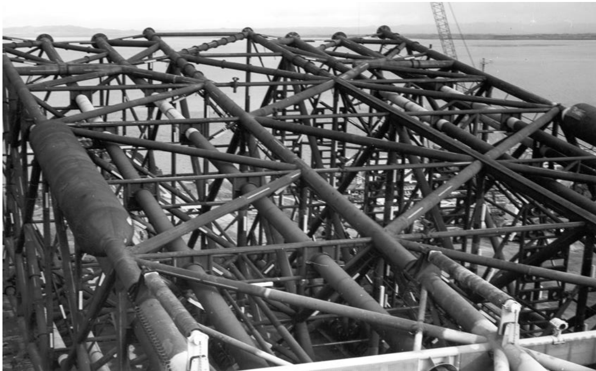
Figure 1-4 Historical image of the Mackerel Steel Piled Jacket prior to installation, showing the complexity of the structure
